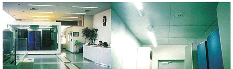
SUPER COMPUTER ROOM PLACE: Ceiling/Wall PURPOSES: Decrease of noise generated from fans to cool computer.
